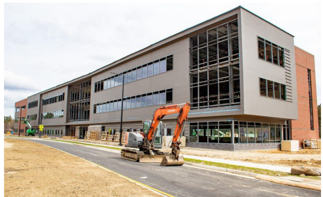
A demonstration lab for the production of green hydrogen fuel will be housed in Building 2, currently under construction, at the Tech Center Research Park in Newport News. Photo courtesy of W.M. Jordan Co.
